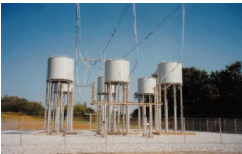
Situated within the right-of-way as a bolt-on installation, six 21-ohm reactors manufactured by Haefely Trench have saved Georgia Power up to $14 million in avoided line installation and station upgrading costs.
